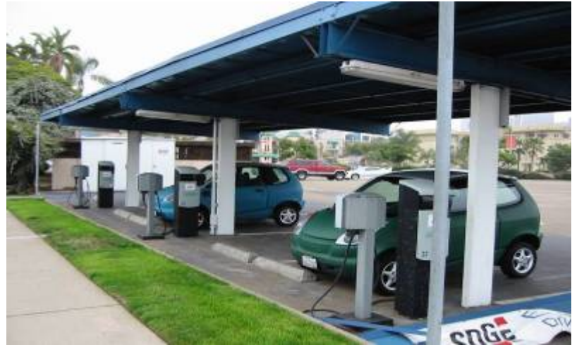
10 kW EV Charging Station
