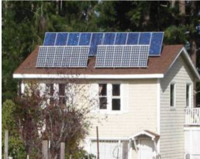
2 kW crystalline modules installed on racks
